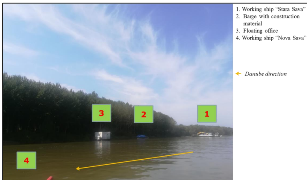
Figure 1 Display of construction sites and auxiliary objects within the Futog critical sector (Futog 2 subsector)
